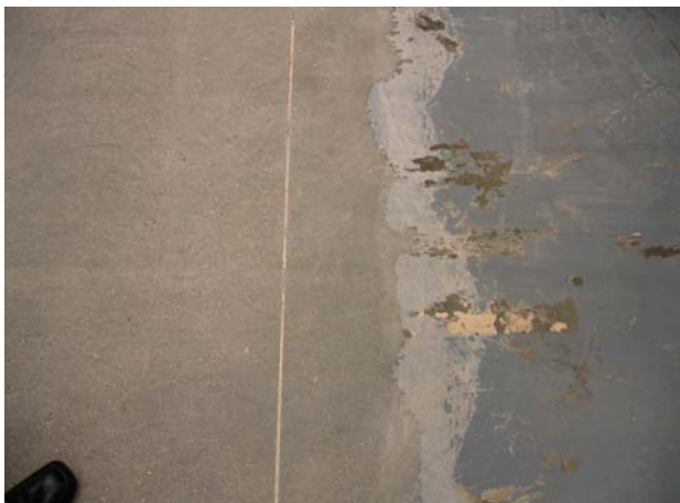
Industrial epoxy coatings being remove using the HTC 800 HD Classic Floor Grinder
